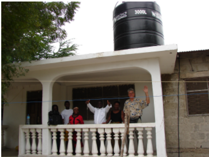
Newly constructed porch serves as tower for the new water tank at home of Estelatus Mtema
